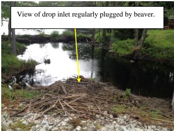
View of plugged drop inlet at sewer line.
