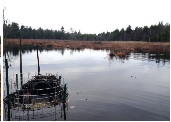
View of protective fence and outlet of the Flexible Pond Leveler at the drop inlet after installation.
