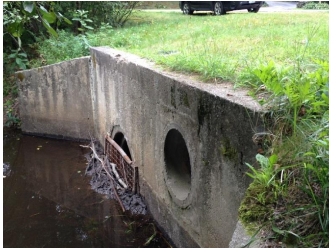
View of beaver damming at a culvert associated with Hanson Drive.
