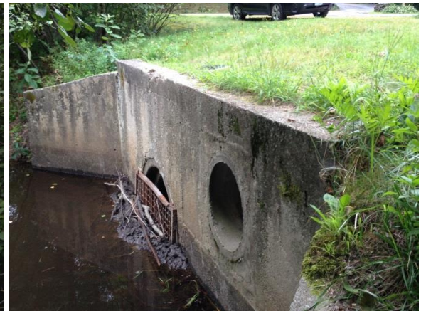
View of culvert damming at Hanson Drive.
