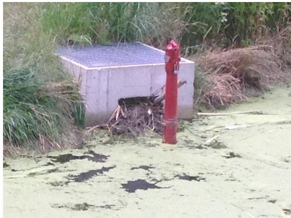
View of plugged inlet.
