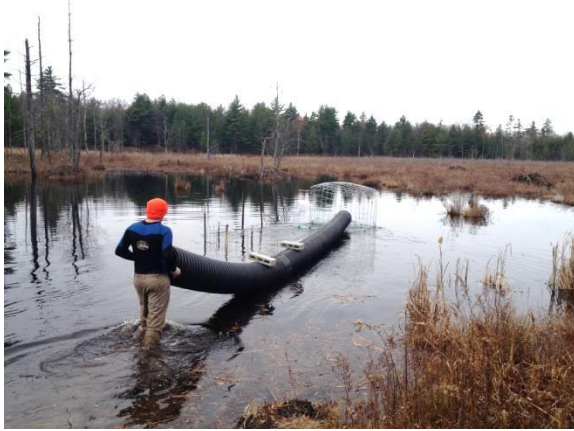
View of Constructed Flexible Pond Leveler just prior to installation at the drop inlet.
