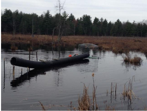
View of Flexible Pond Leveler prior to submersion.
