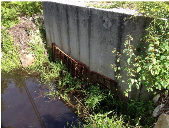
View of plugged culverts at Continental Blvd.
