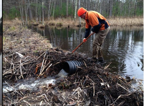
View of pipe outlet installed in beaver dam.
