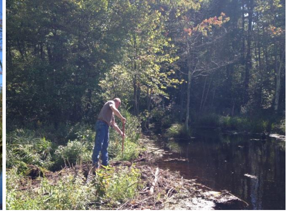
View of large beaver dam and area of old underwater culverts and associated carriage road.
